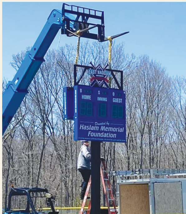
Brian Barzee of Northeast Scoreboards in East Haddam works on installing scoreboards donated by the Haslam Memorial Foundation. The project finished just in time for the April 30 Opening Day of East Haddam/Moodus Little League.
